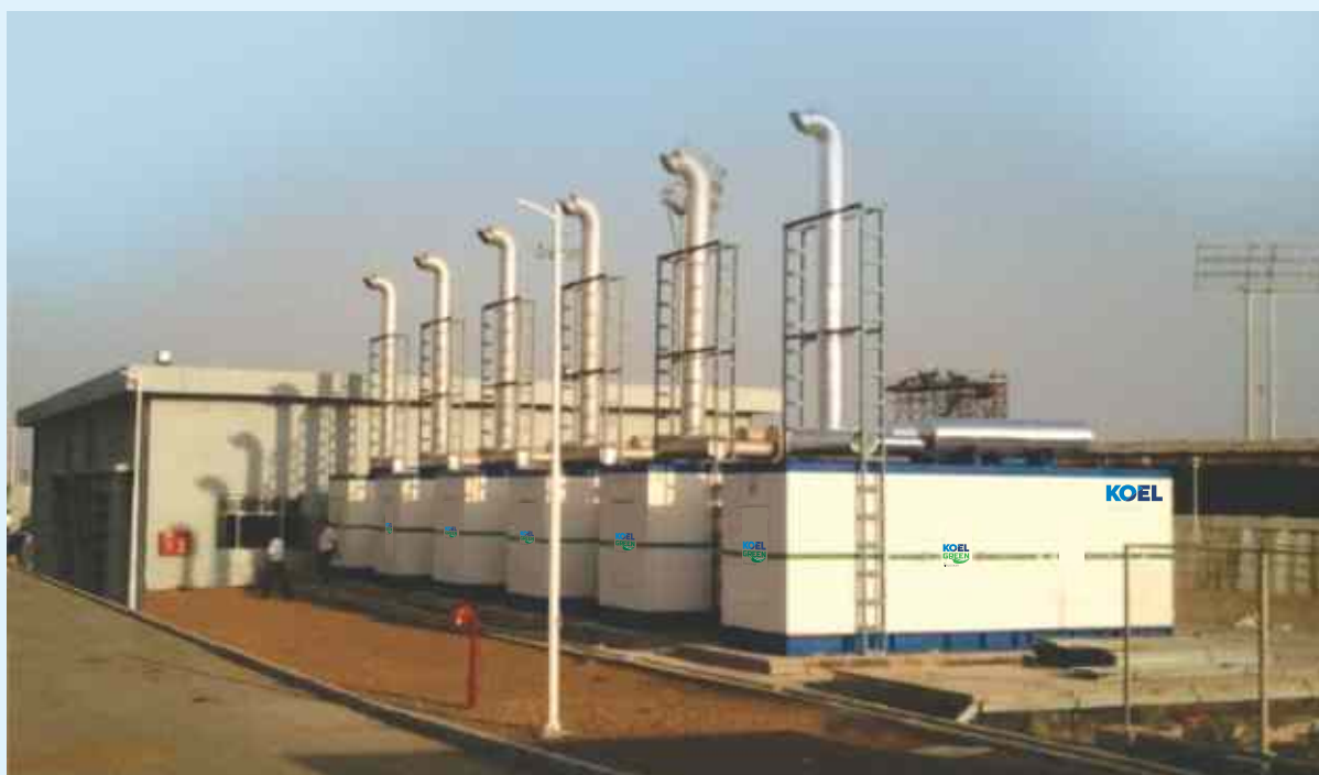
MODERN SPORTS COMPLEX 6 x 600 kVA Typical installation
